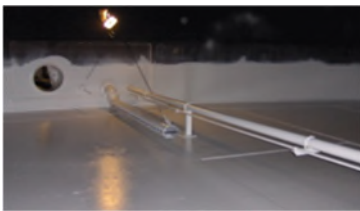
Interior crude oil storage tank
